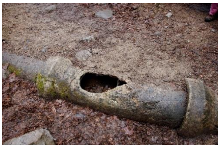
Runoff pipe in disrepair. Source: Tracy Lee Carroll
